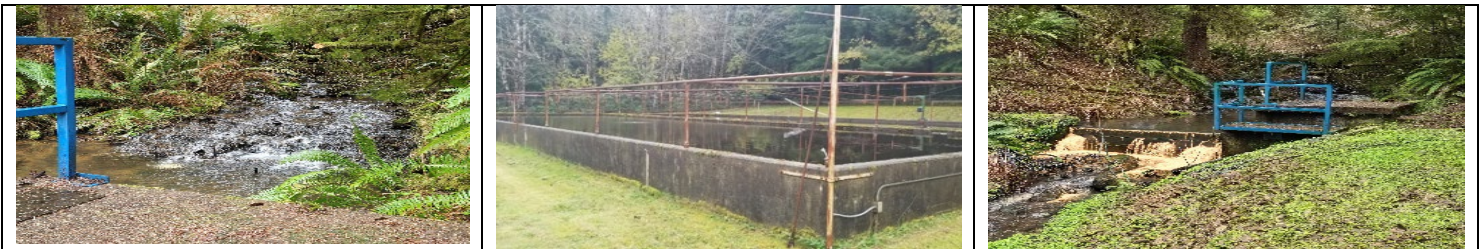
Our slow sand treatment plant (shown above) on Akerstedt (entry point A) receives its water from John Day Creek, also known as Big Fat Buck, and a small tributary to the John Day Creek, locally known as Little Fat Buck.
